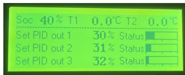
Outputs 1-3 - general settings according to SOC value. battery + output status
